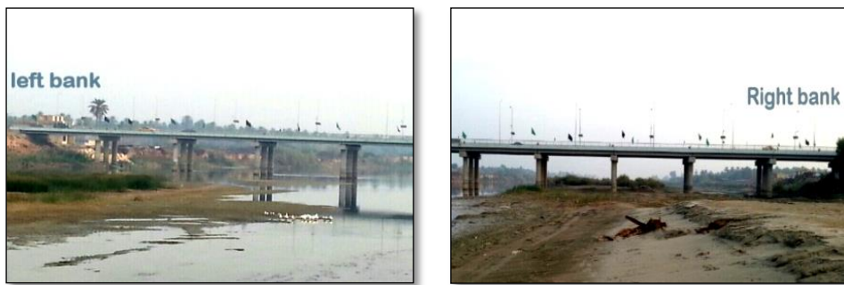
Figure 5: Deposition Upstream the Bridge
